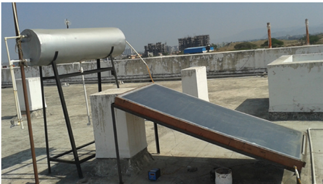
Fig. 4. Photo of solar concrete collector with insulated storage tank.
