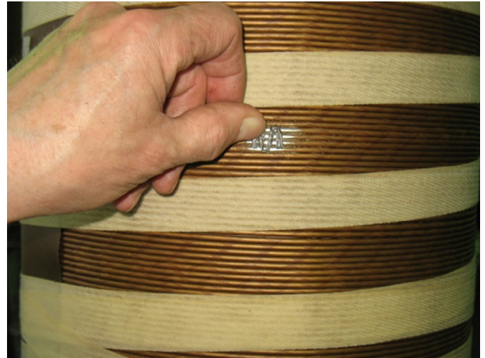
Fig. 5. View of defect “turn to turn short circuit” type made in HV winding.
